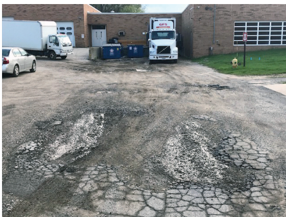
The deteriorating service loop at the high school is scheduled to be resurfaced this summer.
